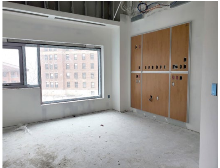
A “walled” patient room showing the headwall that will include integrated bedside technology.
